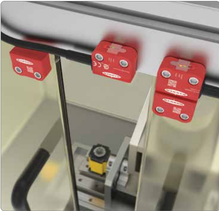
Non-contact switch on a sliding door
