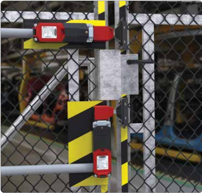
Locking switches on large gate
